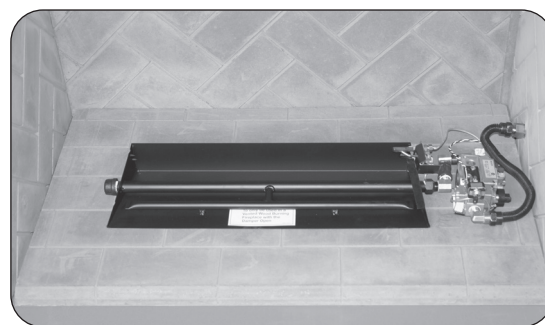
Fig. 16-2 Center burner in fireplace
